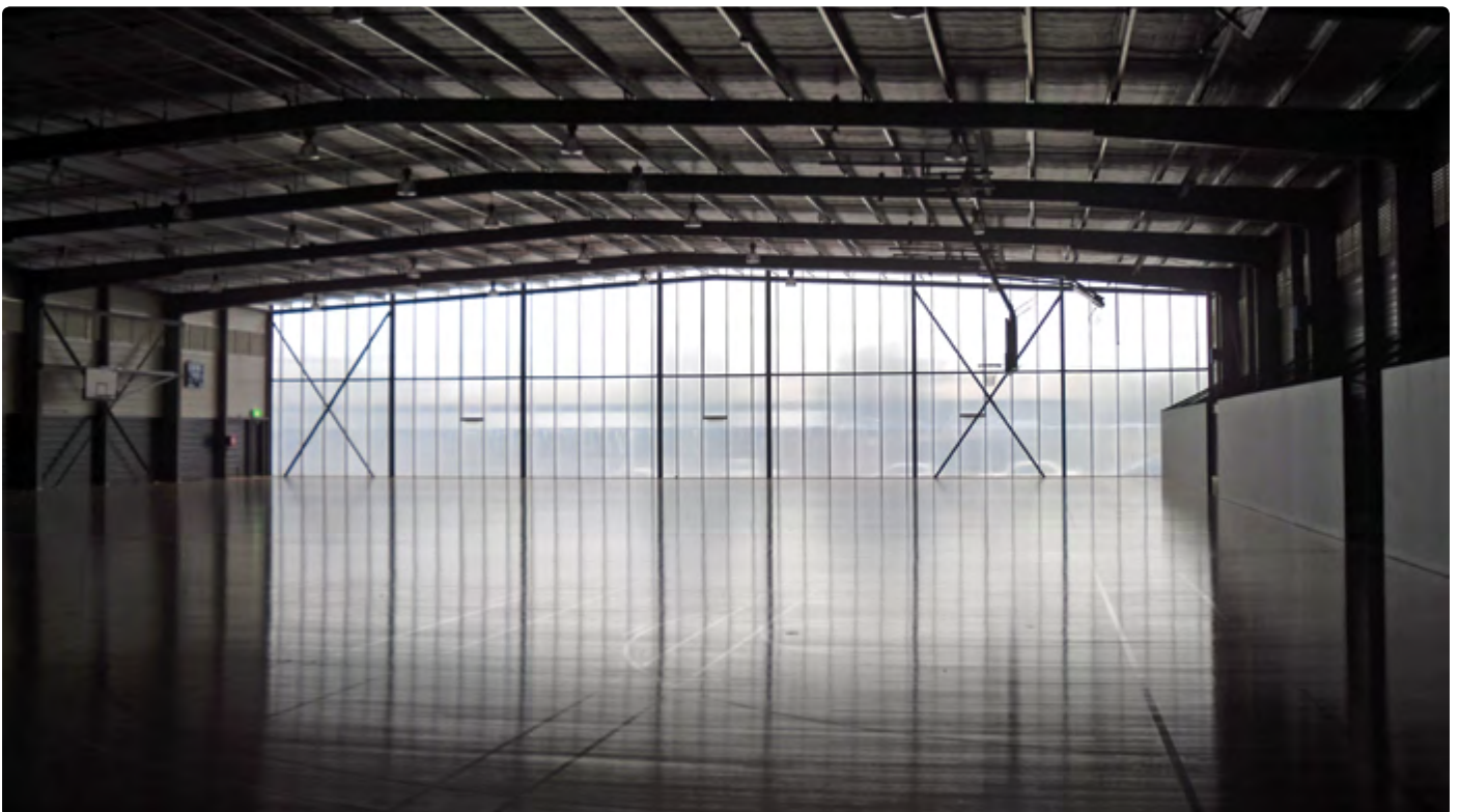
Whitten Oval Community Sports Hall, Australia | Architect: Peddle Thorp | Application: Curtain Wall - 370 sqm | SUNPAL® Type: Solar Ice 18mm
